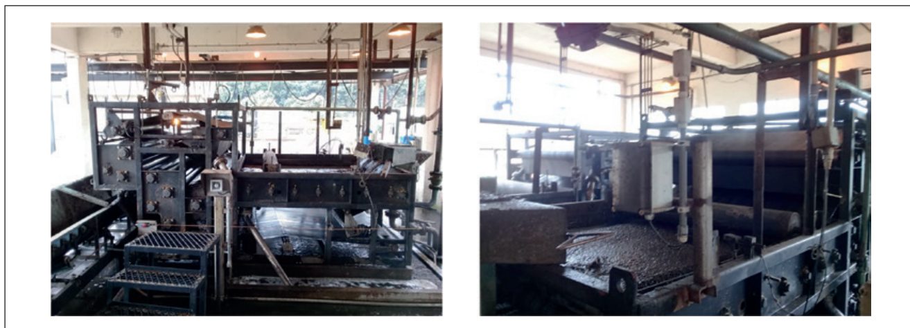
Figure 1: Photos of belt presses for dewatering secondary sludge.
