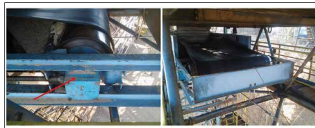
Figure 2. Chip conveyor belt return roller housing
